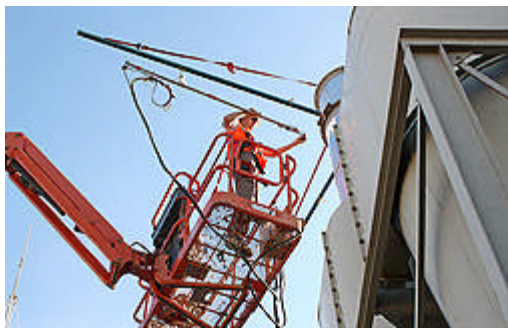
Standing in a manlift basket about 30 feet off the ground, agricultural engineer Clif Boykin inserts a sampling probe into a cyclone stack at a cotton gin in California.
